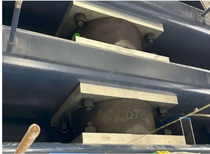
Figure 2: Elastomeric bearing on soil box
