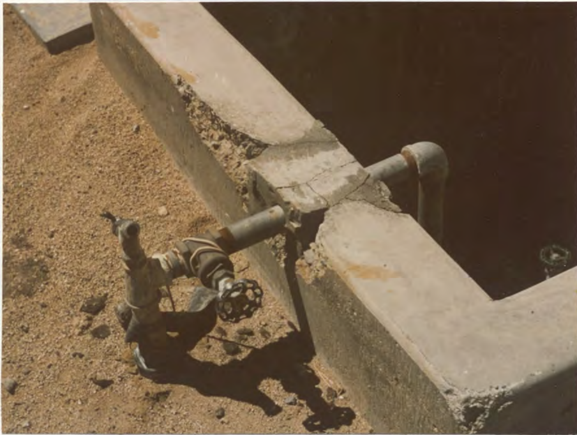
FIGURE 46. Water pipe and concrete retainer wall. The water pipe pulled from the concrete which was patched. Later, however, events have begun to remove the patch.
