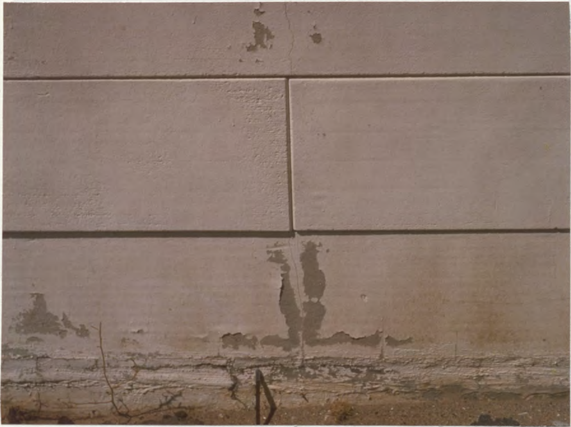
FIGURE 45. Closeup view of machine shop wall showing cracking and grouting along the foundation where the wall shifted about 2 centimeters off the foundation.
