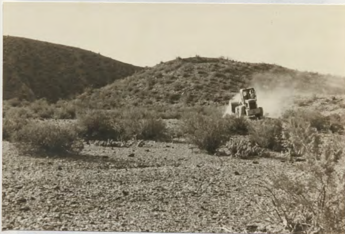
Figure 30. Photograph of trench 11 excavation of the scarp of the Pajarito fault zone (see location on Fig. 31 and Pl. 1). In this area the strike-slip tear fault shows extreme relief across the scarp from conjugate folding, which uplifts the hills across the scarp (left center) and may downdrop the near block by synclinal formation. In this location the scarp is antislope but reverses in other locations (see stereoscopic view in Fig. 31).
