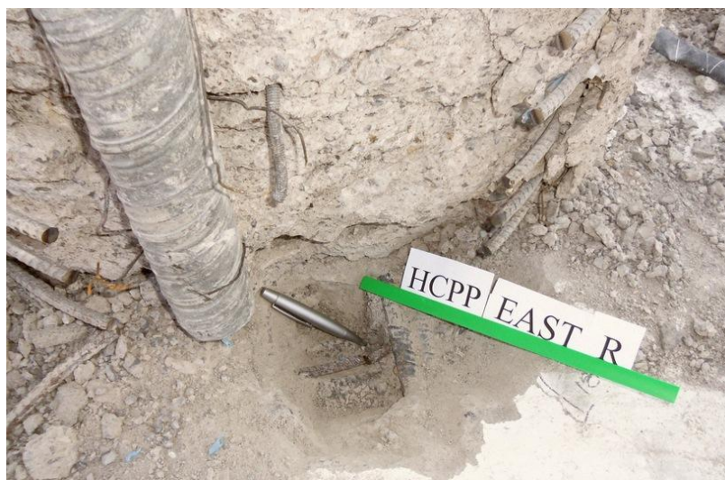
Figure 4-65 Location of fractured bar on the east face of HCPP
