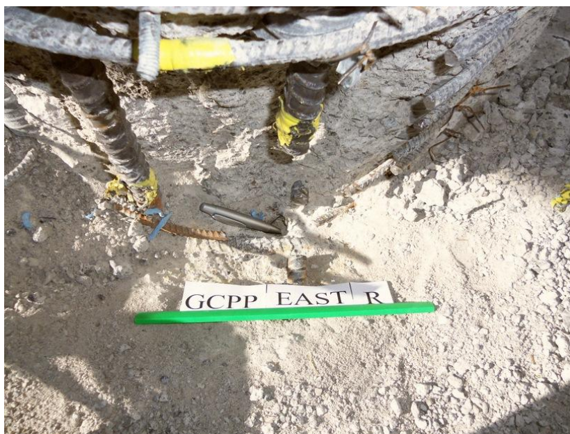
Figure 4-102 Bar fracture location of east face of GCPP
