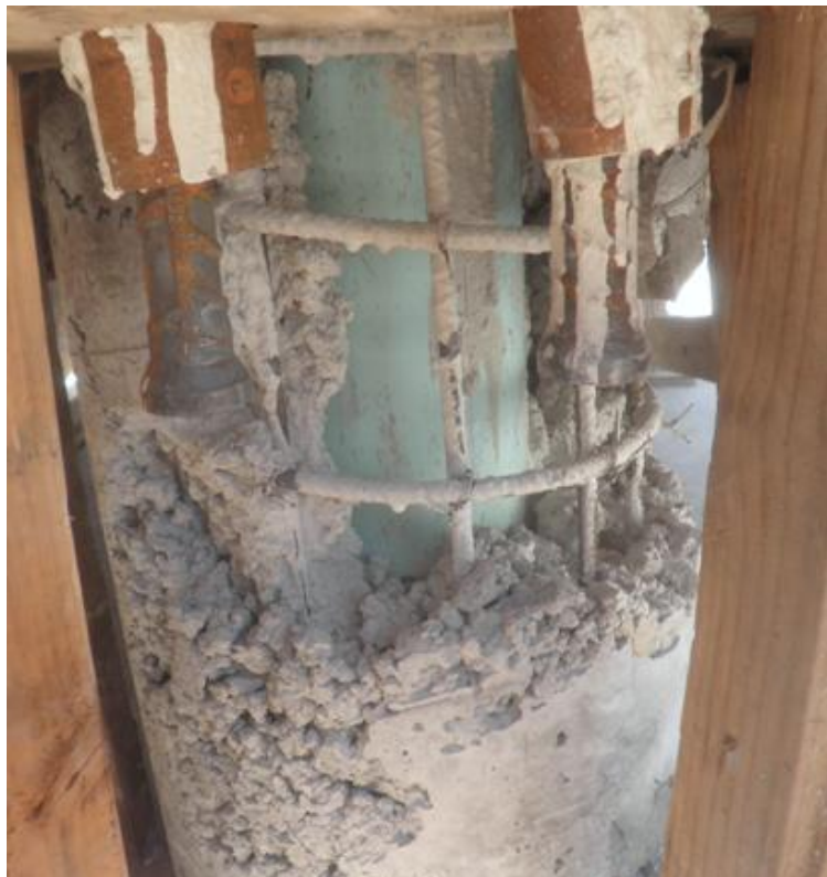
Figure 3-51 Voids found in HCPP coupling region
