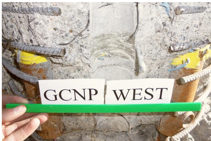
Figure 4-83 Location of removed grouted coupler (center bar west face)
