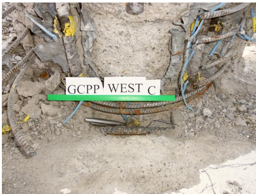
Figure 4-101 Bar fracture location of west face of GCPP
