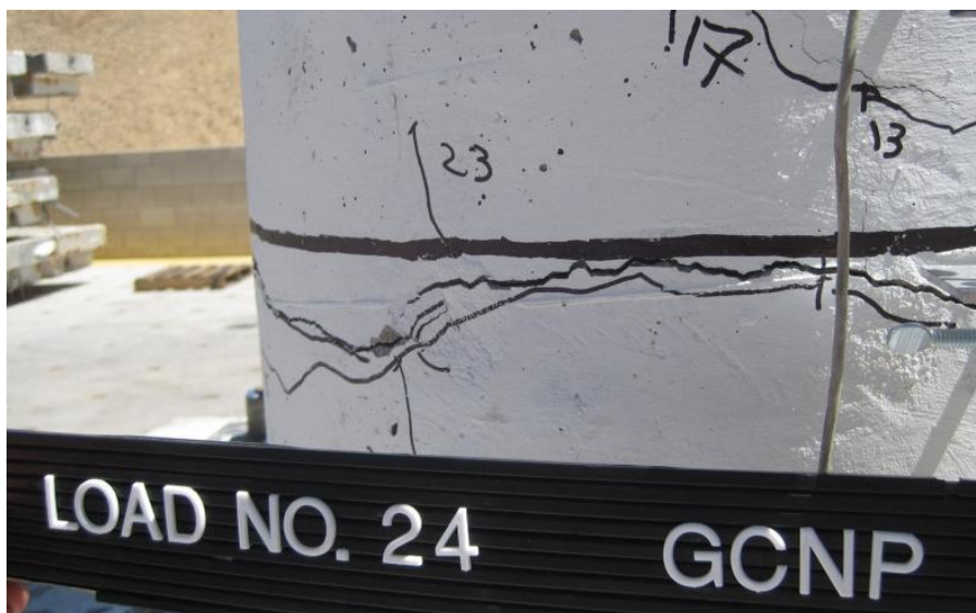
(a) Concentrated crack ( \approx 0.12 in [3 mm]) above coupler region during second push cycle
