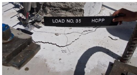
(b) Damage to footing after second push cycle (West face)
