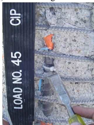
(c) Fractured longitudinal bar on East face
