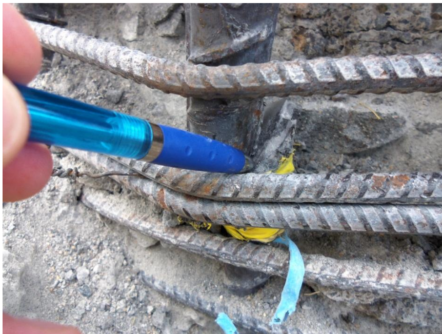
Figure 4-46 Fractured bar located on the east face of HCNP (left bar)
