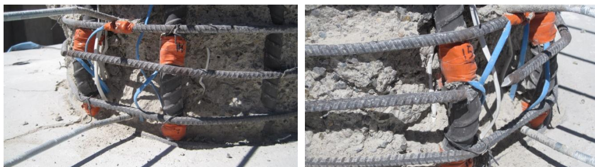
(a) Bar buckling on East face
