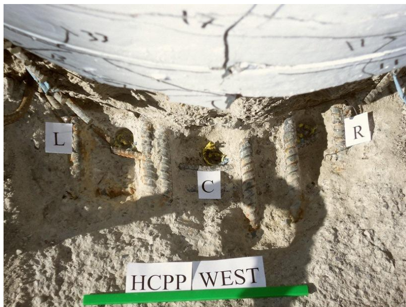
Figure 4-64 Locations of fractured bar on the west face of HCPP
