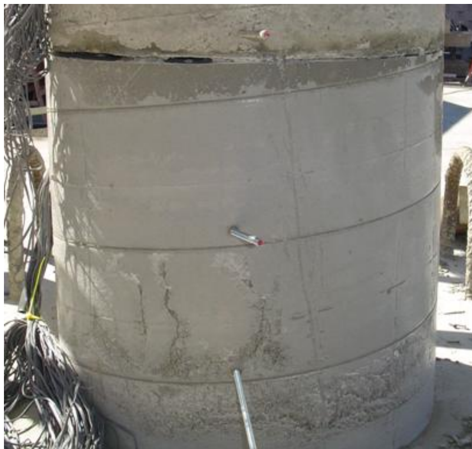
Figure 3-39 Void left from bleed material
