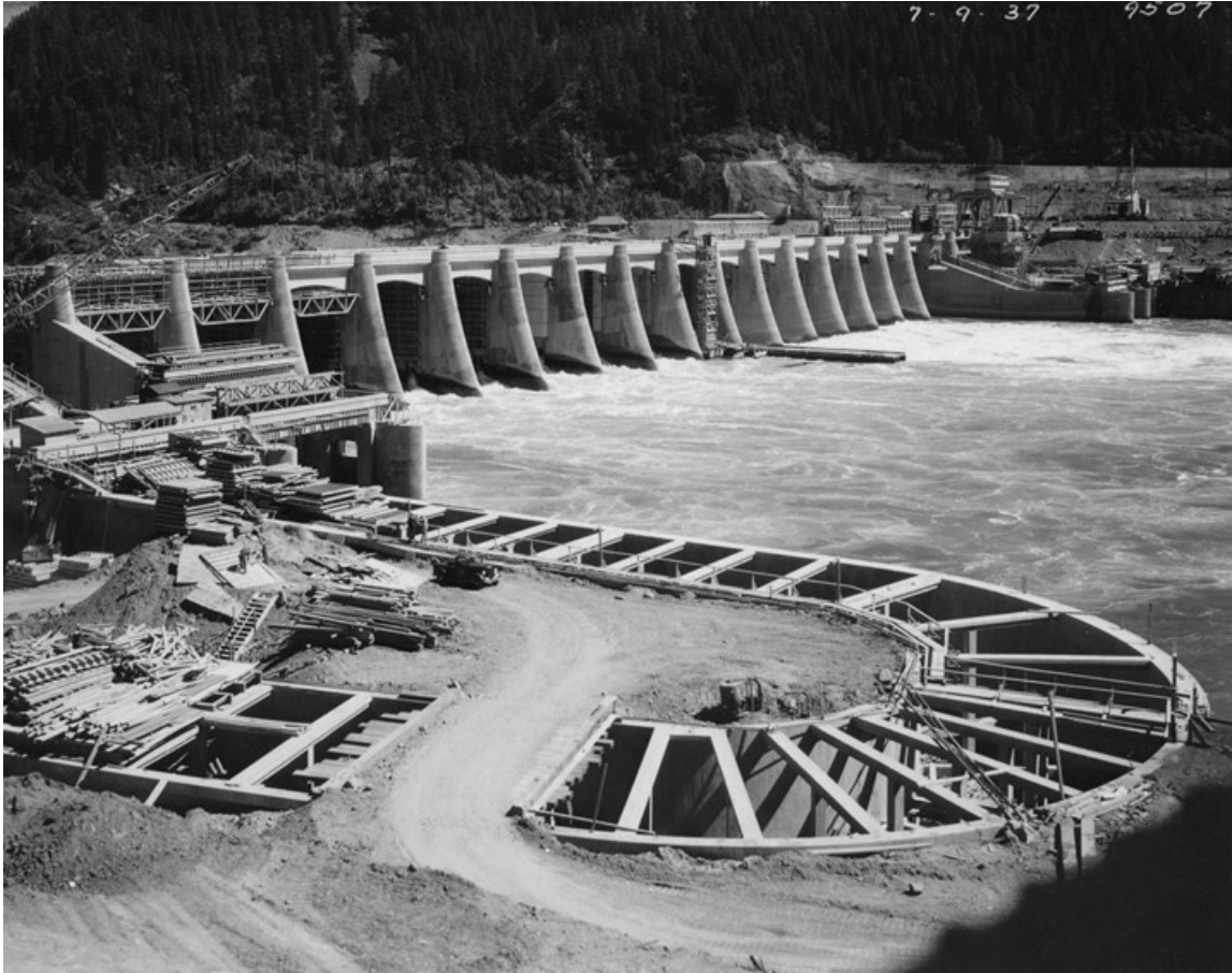
Figure 4-11. Construction of ‘fish ladders’ at Bonneville Dam on the Columbia River, 9 July 1937.
