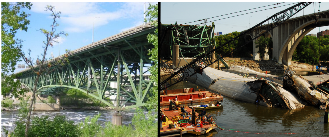
Figure 1.2: I-35W Bridge before and after collapsing [2, 3]
